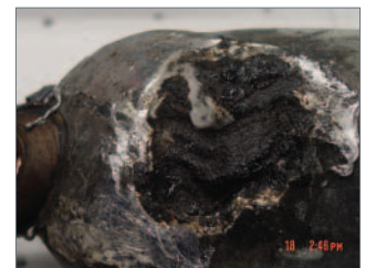
Failure at the lead wipe region of a overhead lead splice.
